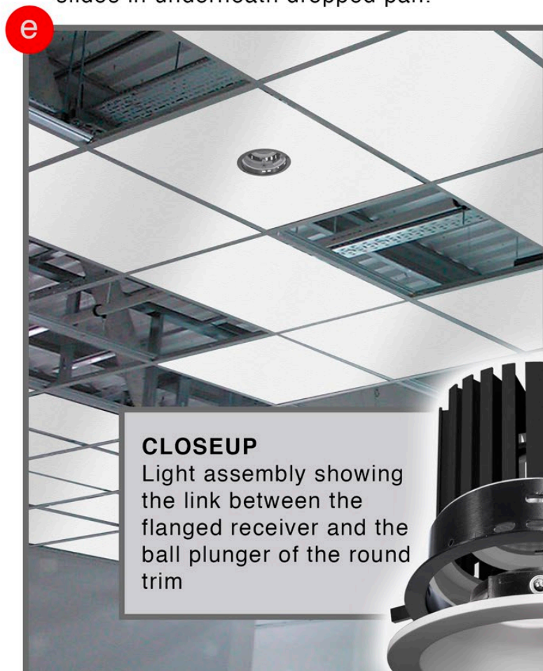
Step E- Use Phillips screwdriver to adjust ceiling clamp that controls tightness of light assembly to dropped pan/ tile. Magnify CLOSEUP to view ceiling clamp
