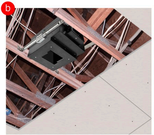
Step B- After housing is secured. Continue drywall install, but leave space for wiring.
